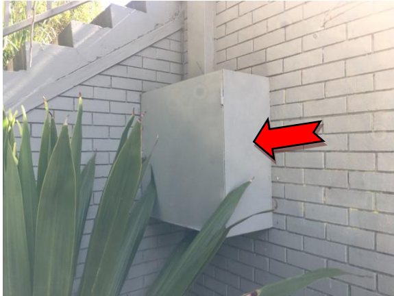
Photo 1. Ground level, exterior, western elevation – suspected asbestos containing bituminous electrical backing board.
