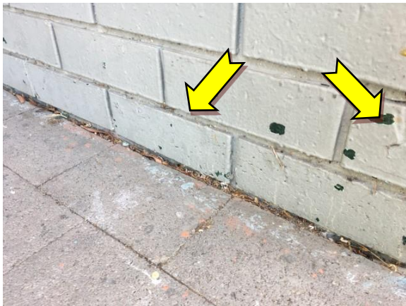
Photo 3. Exterior, throughout walls – suspected lead-containing grey upper and green lower paint systems.
