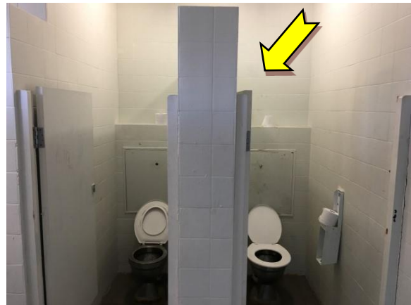
Photo 4. Interior, throughout walls– suspected lead-containing white upper paint systems.
