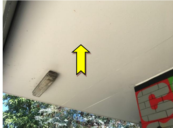
Photo 2. Exterior, throughout awning – suspected lead-containing white upper paint systems.
